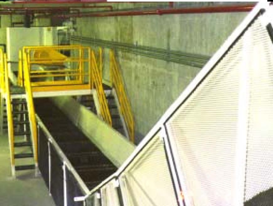
Under-the-floor collector conveyors collect scrap from the presses and discharge it onto branch conveyors for elevation to loading points outside the plant.
