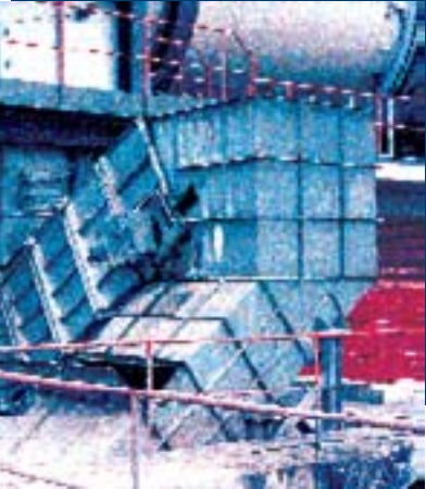
Ash discharge conveyor from 200tpd industrial waste incinerator (Austria)
