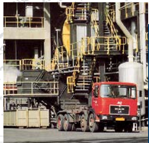
Ash discharge conveyor from 100tpd industrial waste incinerator (The Netherlands)
