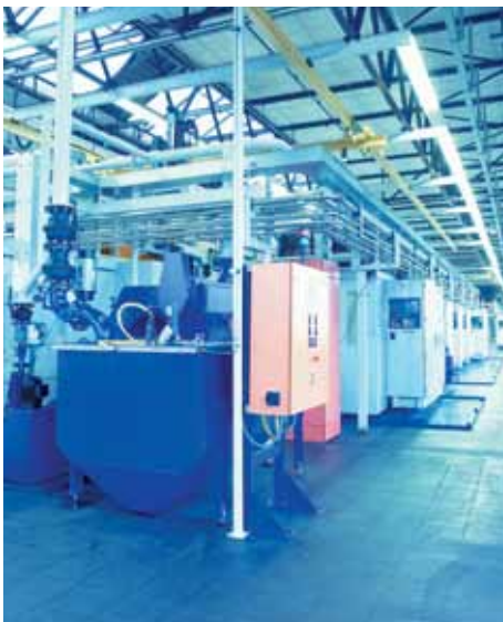
Pump back station for a transfer line
